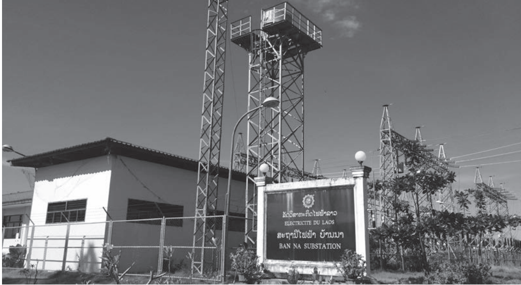
Ban Na Substation in Champasak, Laos.
